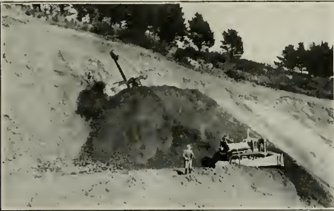
New B-60 "Hidden Power" Ateco Bulldozer Swings into action on the steep slopes of Grizzly Peak Road Extension in Alameda County.
